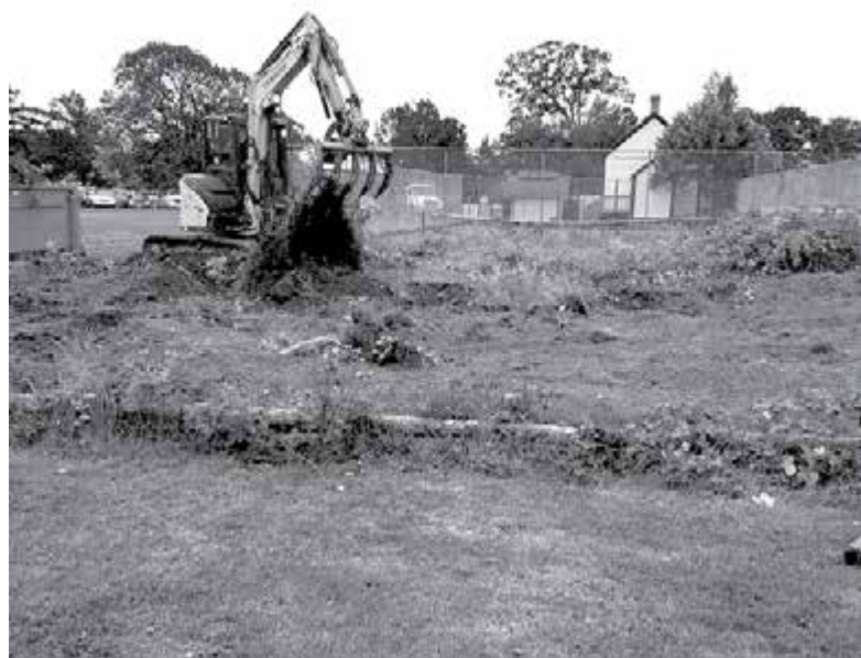
John Ranns operating an excavator, donated by Mr. French, for putting finishing touches on garden site. Shelly Donaldson photo
