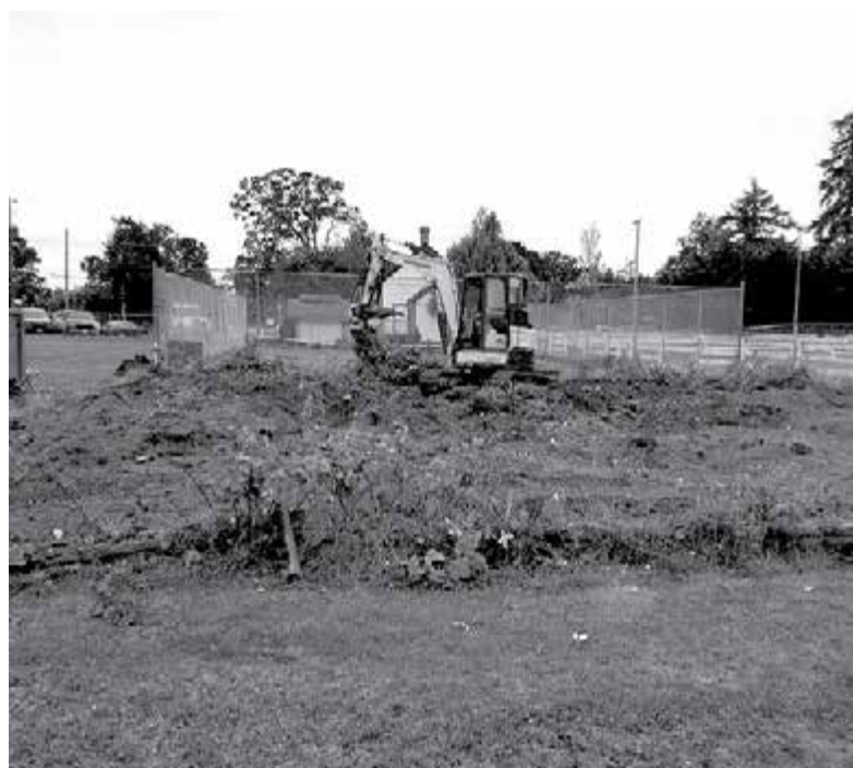
Dan French of French Enterprises donating time, staff and equipment to excavate the four-foot high bramble jungle and rotten beams covering the garden site. Brent Donaldson photo
